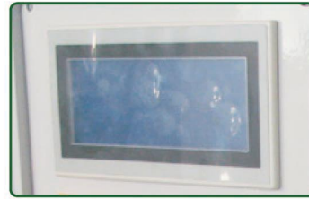
PLC control touch screen
