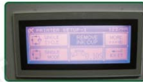
PLC touch screen panel
