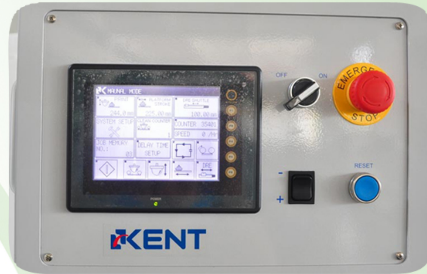
PLC touch screen control panel
